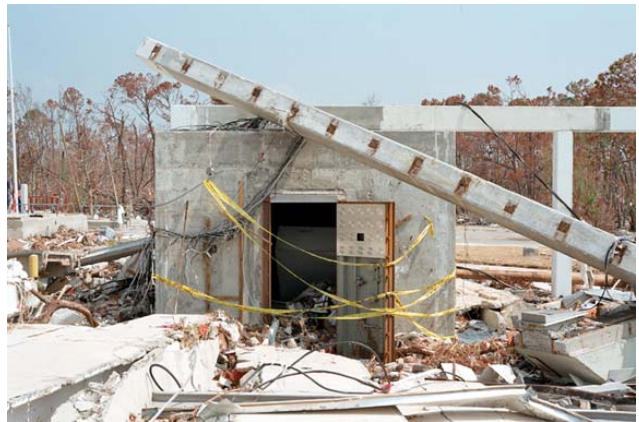
Vault is all that remains of bank in Bay St. Louis, Mississippi.
